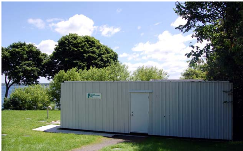
View of compact MBR Wastewater Treatment Plant with view of St. Lawrence River
