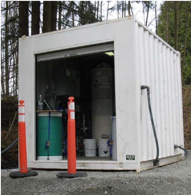
“IRON STOPPER” Containerized Treatment System, including the “DEFERUM™” hydro-automatic filter
