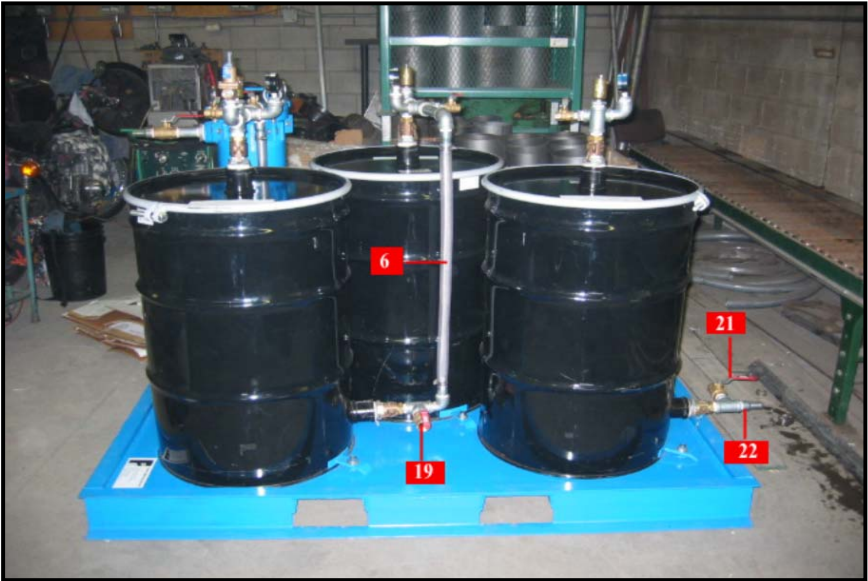
Photograph 3 – 5 GPM Pump & Treat System (Third View)
