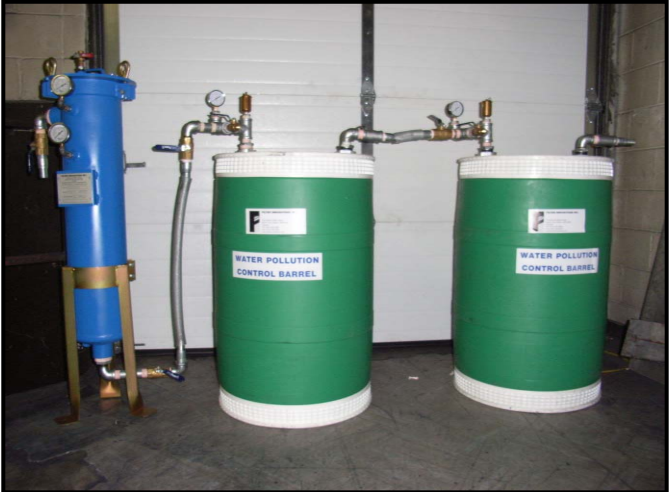
Photograph 1.0 – Pump and treat system
