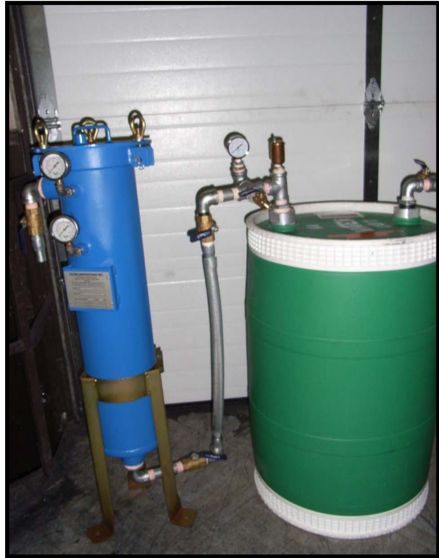
Photograph 3.0 – Bag filter and carbon drum
