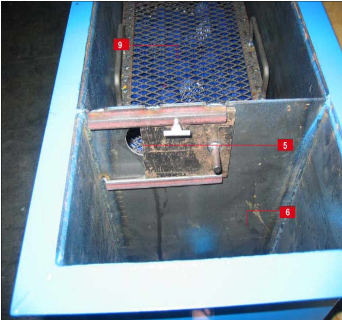
Photograph 3 – Oil/Water Separator (Alternate Top View)
