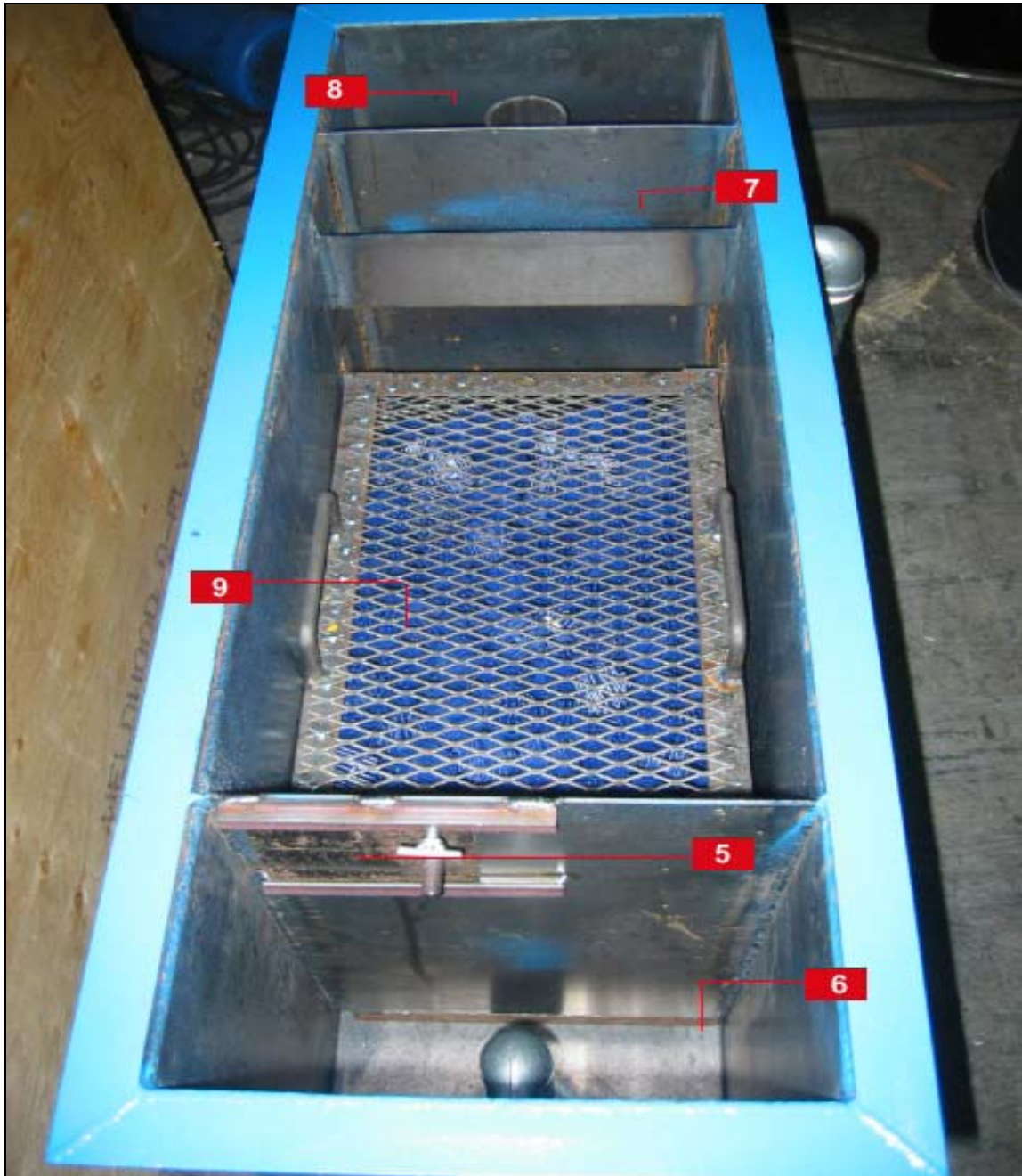
Photograph 2 – Oil/Water Separator (Top View)
